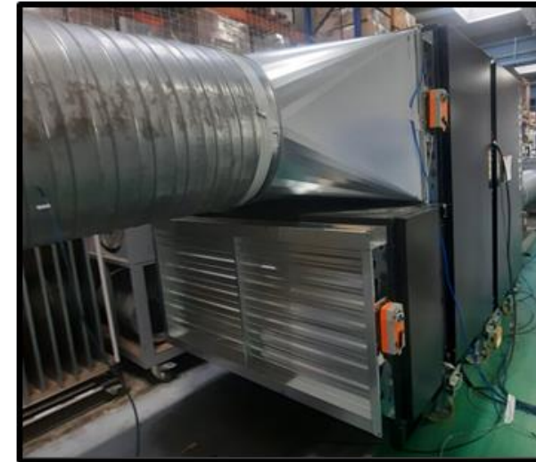
Tests on real AHU (or Field tests)
